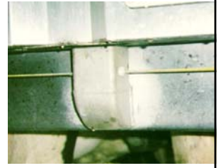
Coated Cable in parlor
